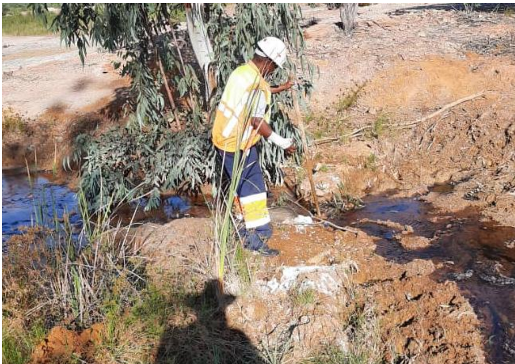
Figure 7 : Image showing the process that assists in neutralising the acidic water before being discharged into Deka Rive)
