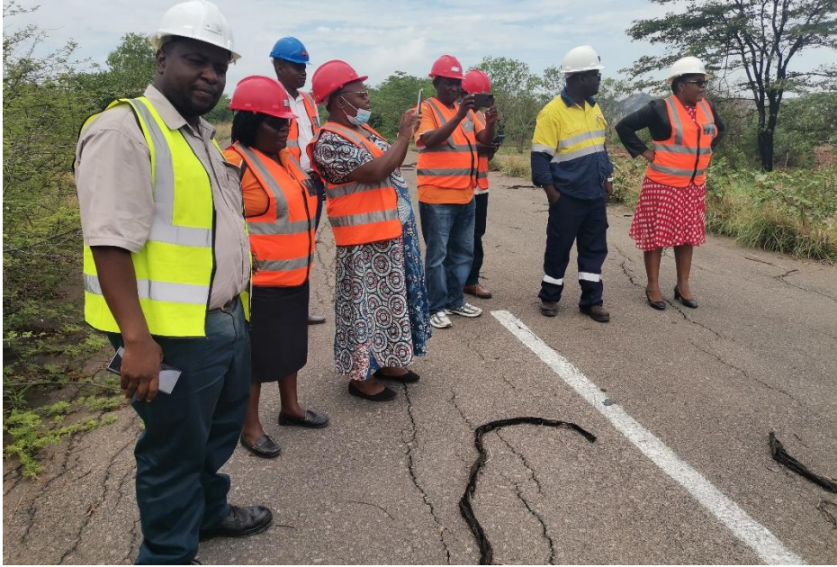
Figure 6: ZHRC and HCCL Management viewing cracked road due to underground coal fires
