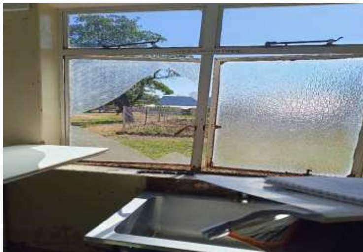
Figure 2 Showing broken windows in the female ward
