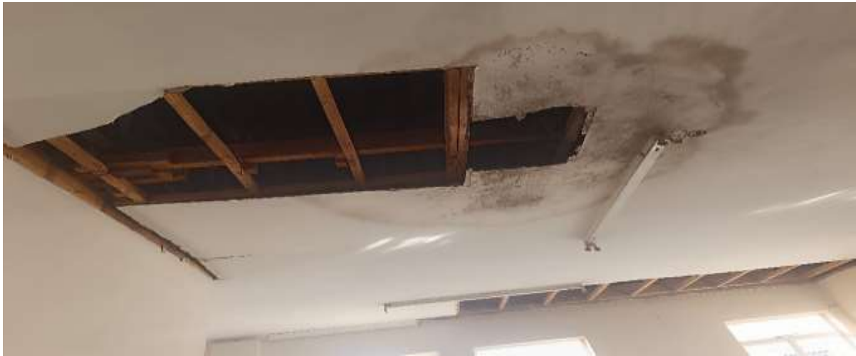
Figure 1 Picture showing detached ceiling
